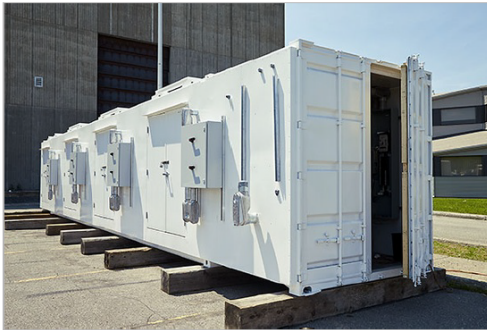
Large-capacity energy storage system prototype
